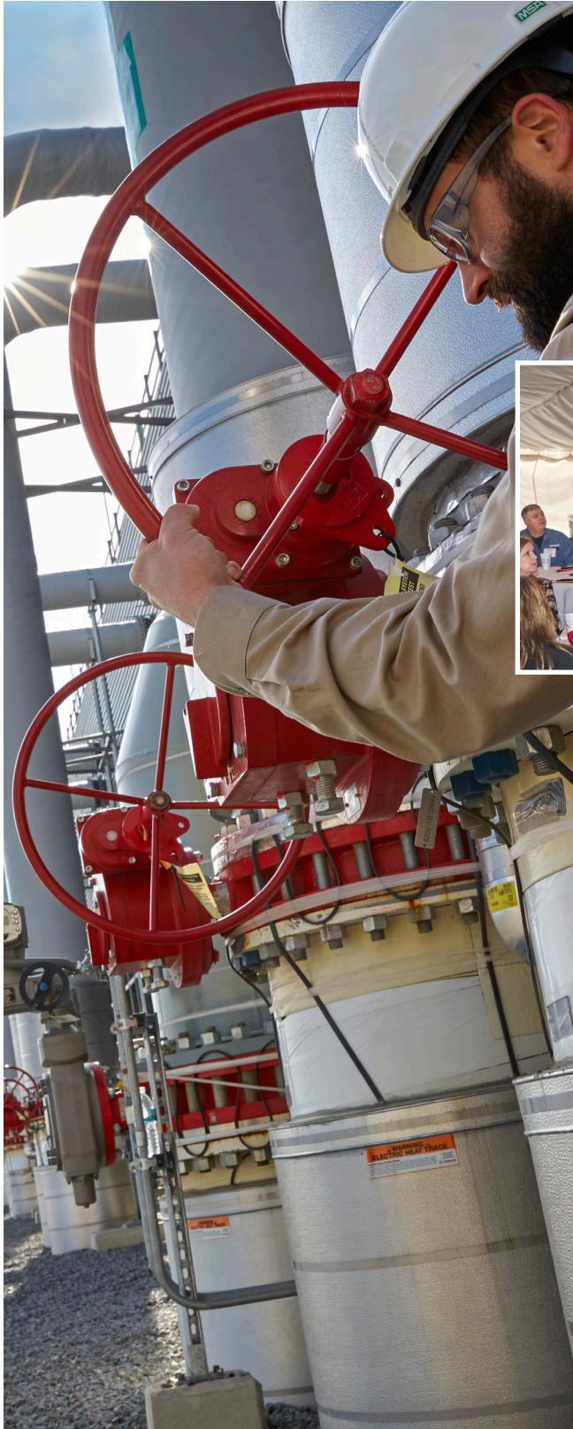
Employees at the Tenaska Westmoreland Generating Station near Smithton, Pennsylvania, regularly monitor equipment to ensure the plant is operating safely and efficiently.
